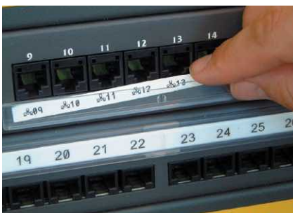
Punch block & patch panel labels
